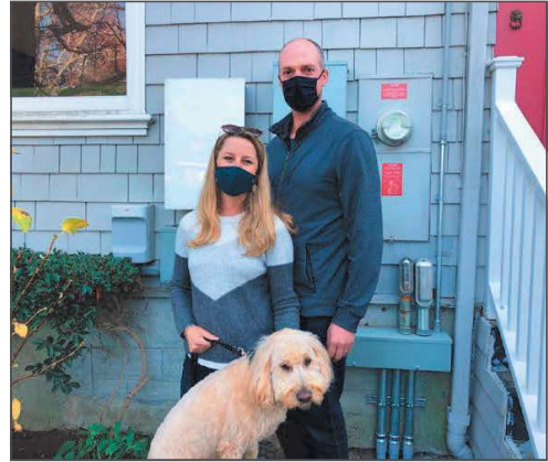
Ben and Cortney Allen with Oakley in front of their tastefully mounted solar power control panels.
